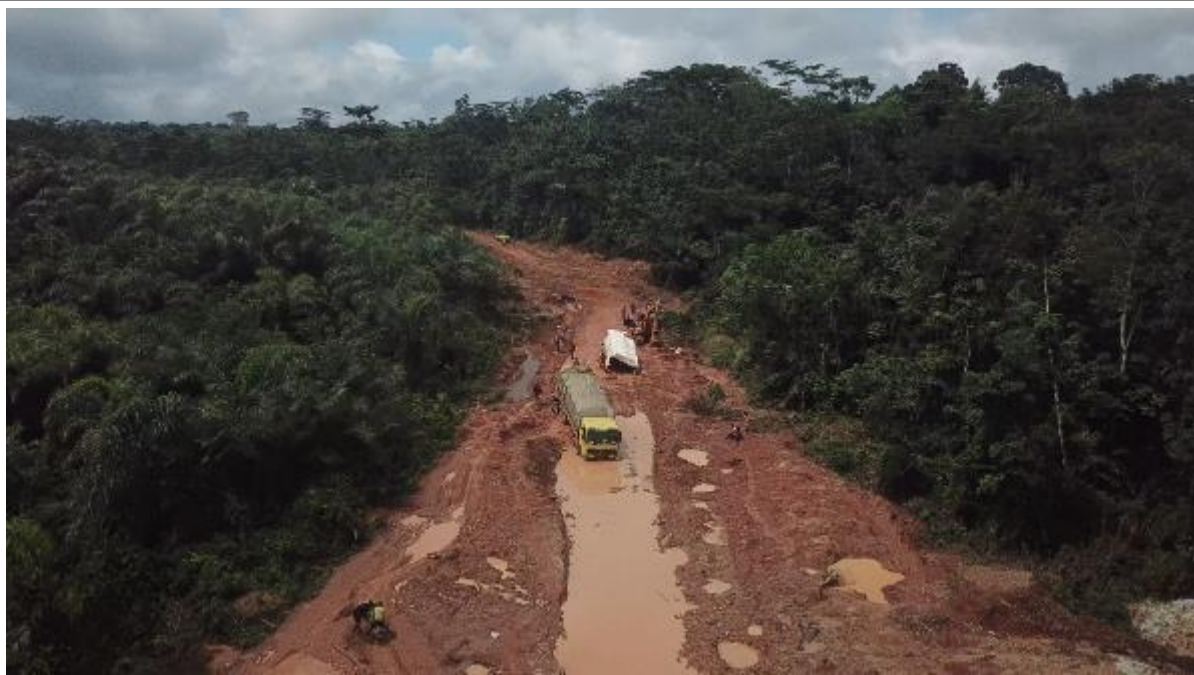
Figure 3-2 Typical development of critical sections along the Road in the rainy season (Source: Earthtime, September 2018)
